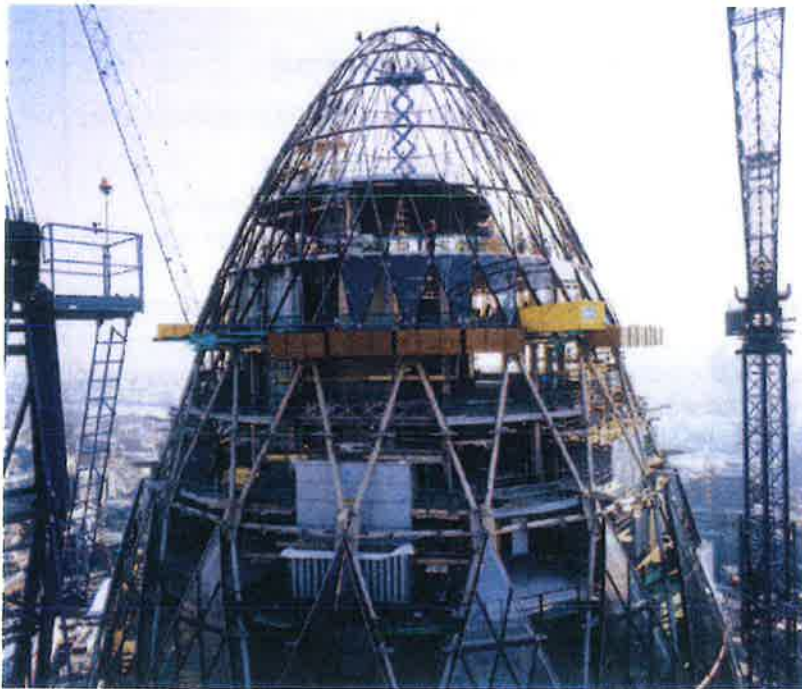
CDM Regulations protect workers from the construction to demolition of large and complex structures.
