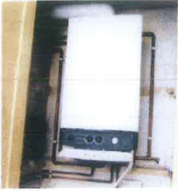
Pipework to boiler
