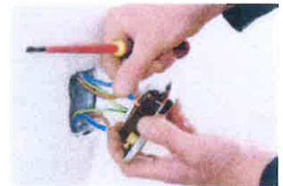
Electricity cables, switches and socket
